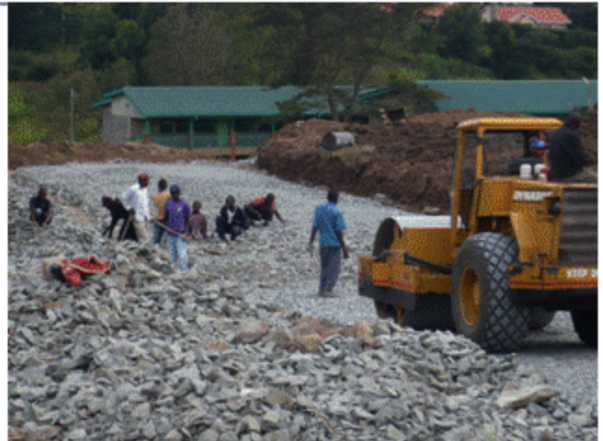
Construction in progress of the access road that connects the school and the Parish
